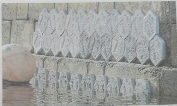
The new tiles made out of recycled quarry waste have been installed in Falmouth Harbour to promote marine life
